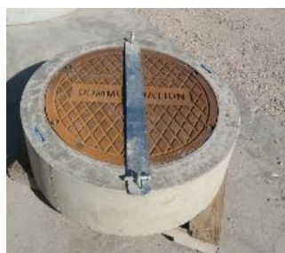
Fig 2: Padlocked manhole security system
